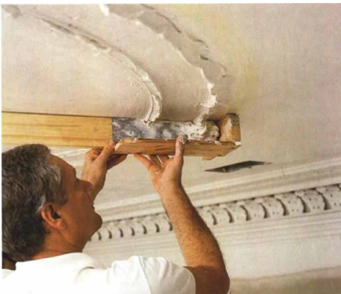
Flaharty uses a template to run the plain molding of the stair-hall medallion. A well catches falling plaster as the template is pivoted on a screw at the center of the medallion.
