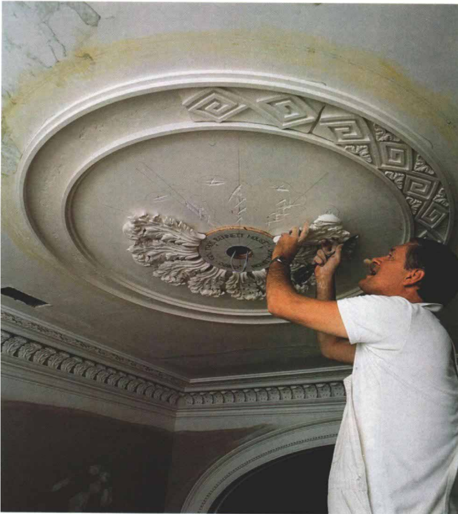
A plywood stop allows precise placement of the acanthus-leaf cluster. Before attaching the ornaments, Flaharty marked guidelines with a shop-made protractor, then scratched along the lines to give the plaster adhesive a better grip. The ornament is then painted with a bonding agent and the ceiling is misted with water. These steps prevent the adhesive from setting too quickly.
