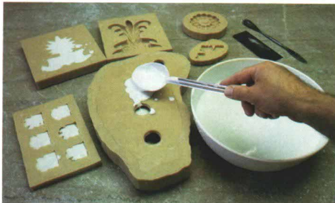
Flaharty spoons casting plaster into the two-part urethane mold of the stair-hall medallion. He's already poured a gang mold and single mold for parlor ornaments.
